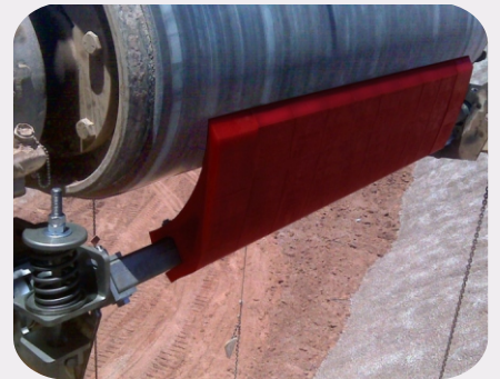
Skalper MDX with Spring Shoc tensioner and dual durometer blades installed on this 72" wide ore handling conveyor system.
